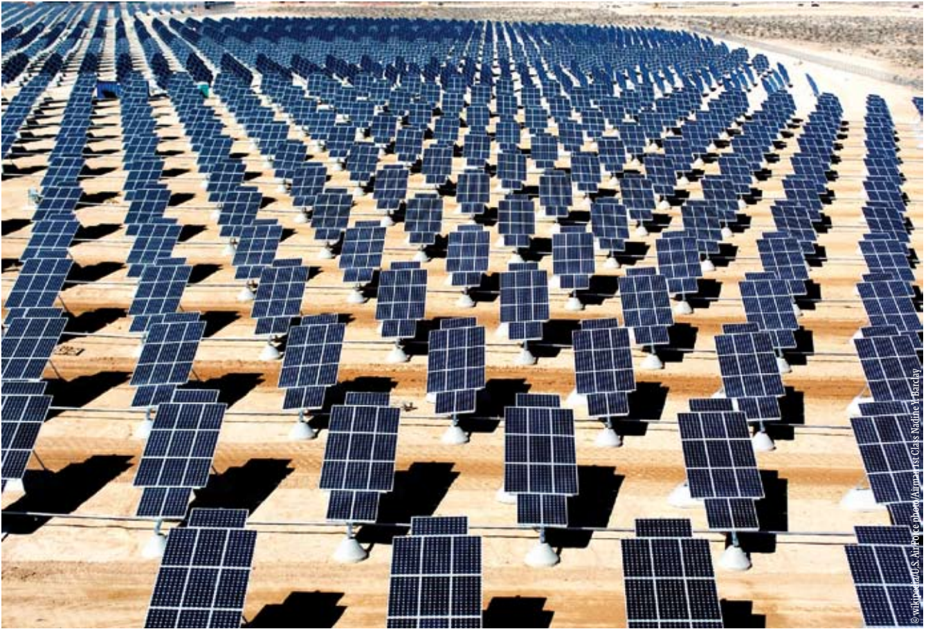
70,000 solar panels configured to form a giant photovoltaic array collecting solar energy at the Nellis Air Force Base, Nevada
